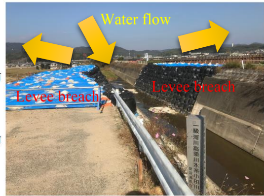
Fig. 2 Levee breach at Oda River in Mabi City
